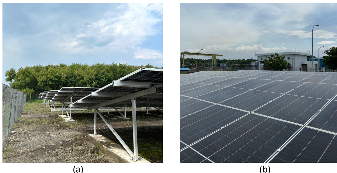
Fig. 10. Actual field condition of the PV system: (a) northern-side view, (b) southern-side view, showing open-site installation with minimal shading from surrounding trees and nearby structures
